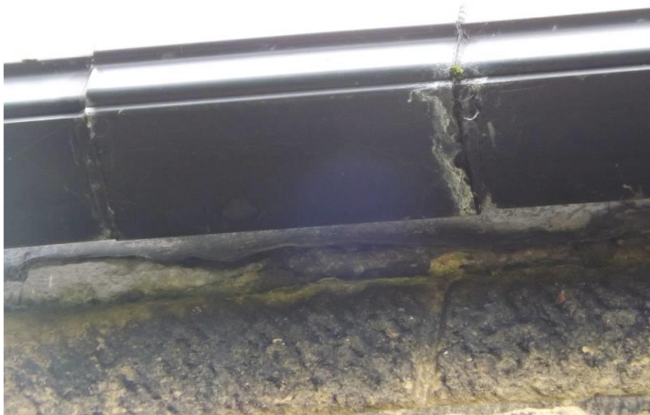
Leaking gutter joint
