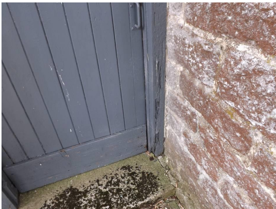
Rot to outside WC door frame
