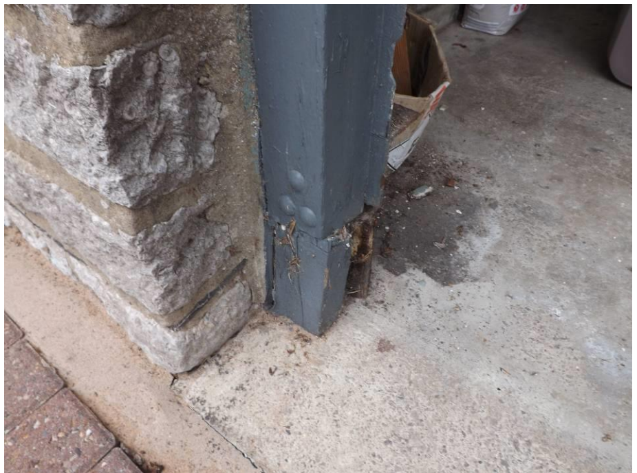
Rot to garage door frame
