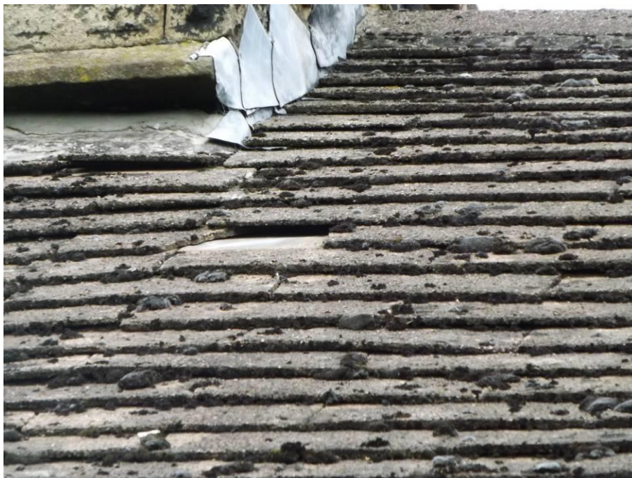
Slipped roof tile
