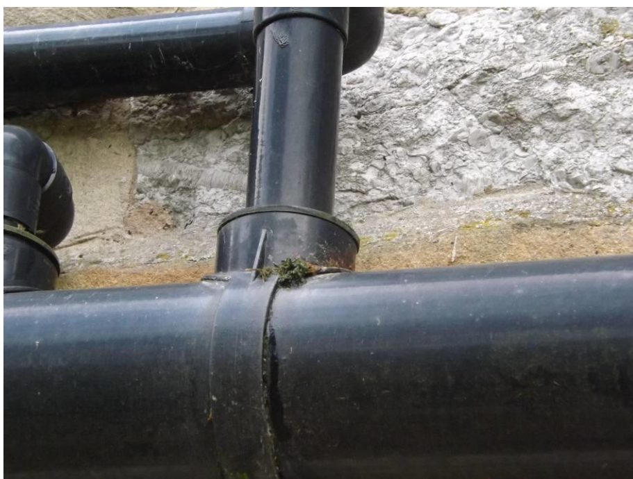
Leaking boss connected waste pipe
