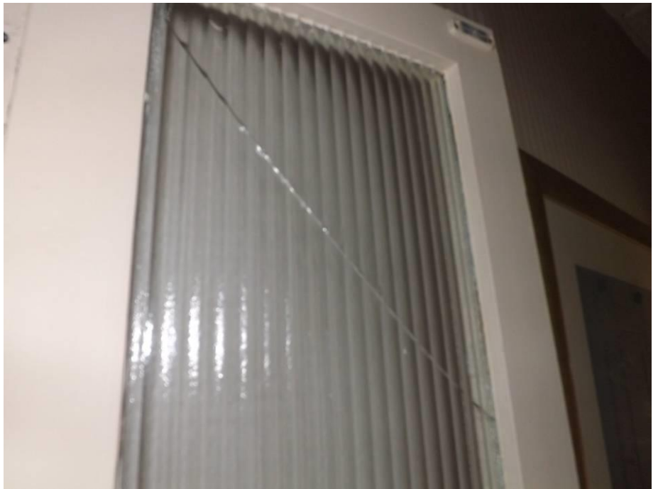
Cracked internal door glazing
