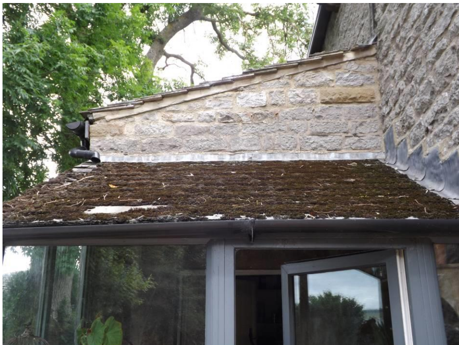
Moss on entrance porch roof
