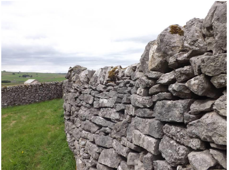
Deflected boundary wall
