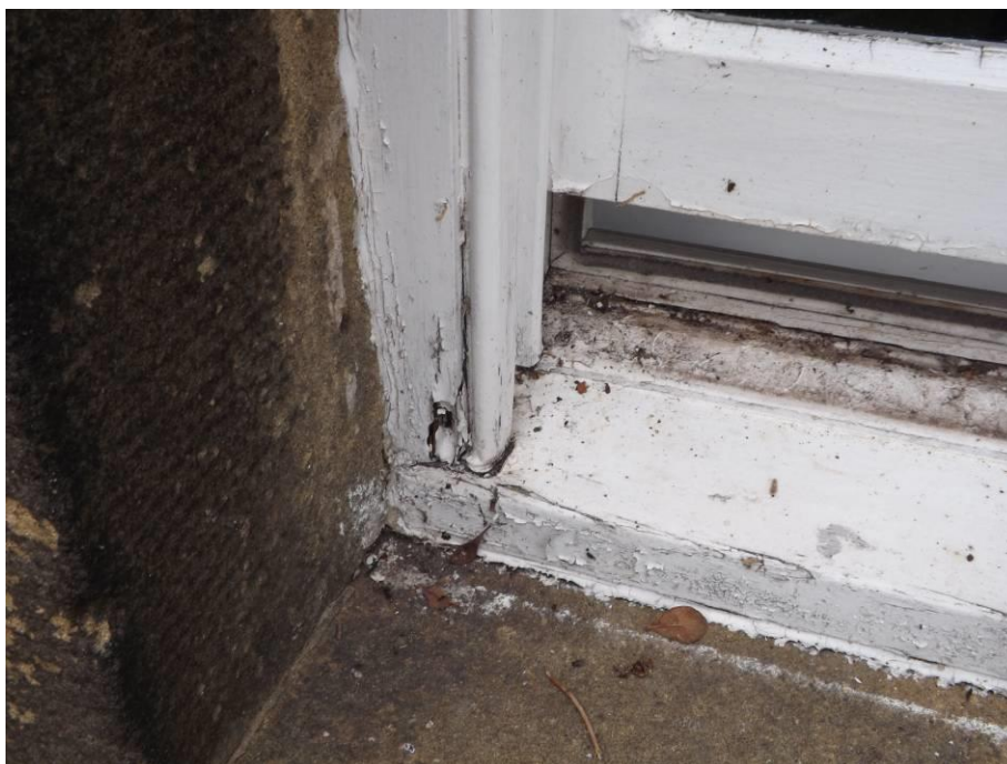
Rot to window joinery
