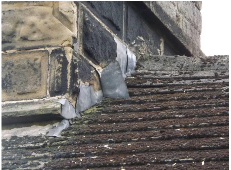
Loose chimney stack flashing
